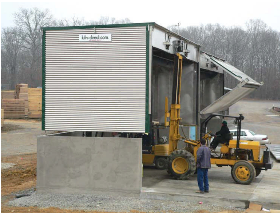
Cline Lumber was able to increase the capacity of the Kiln-direct dry kilns by installing them on 6-foot-high concrete walls; photo taken during the installation shows three forklifts being used to set the modular structures on the raised foundations.
